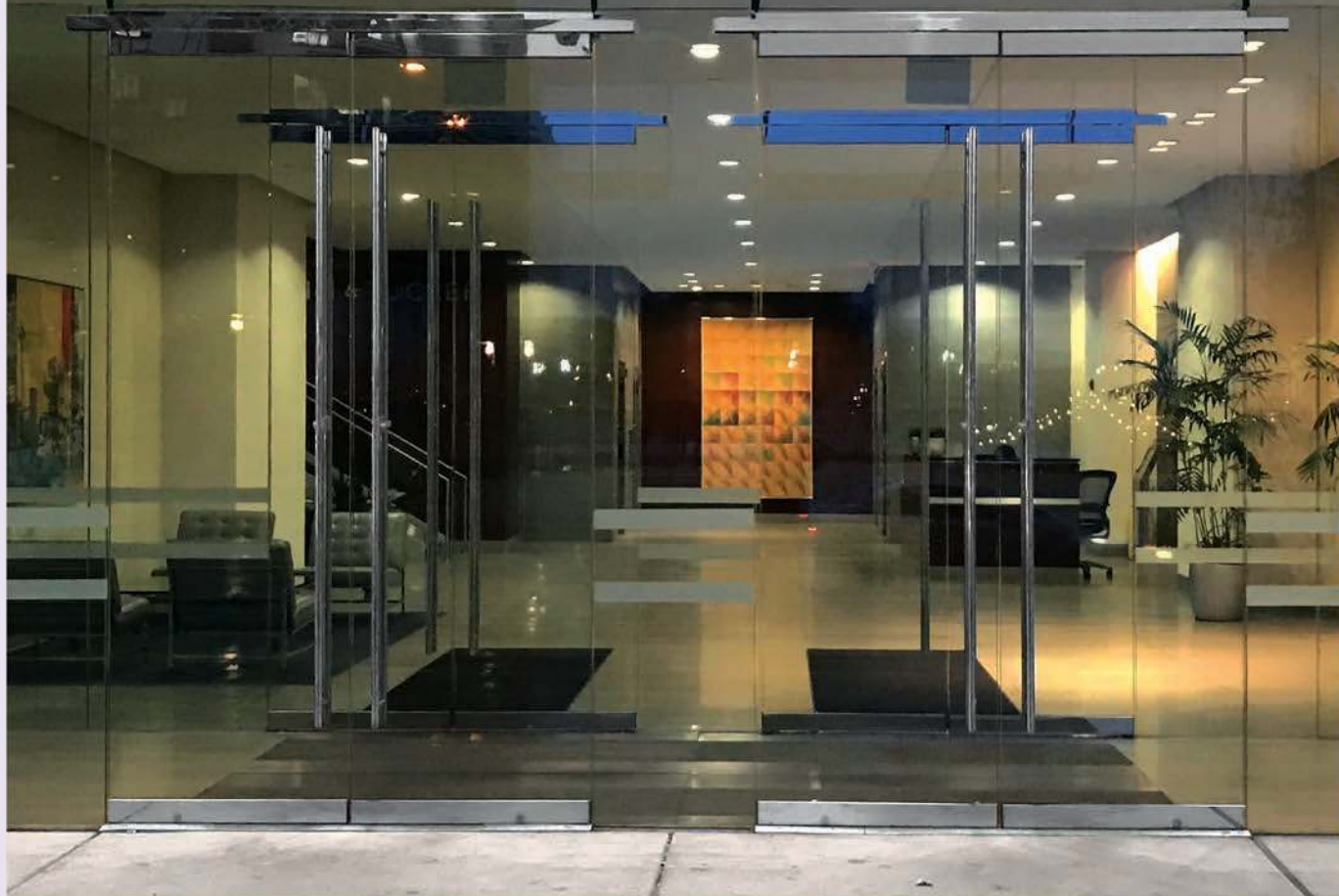
Entrance Doors with Stainless Steel Floating Headers
